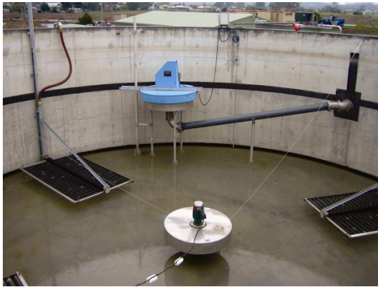
Figure 5: Internal components of the SBR Tank showing Mixer, Aerators and Decant Mechanism
